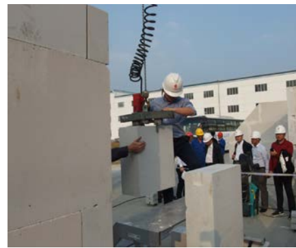
First-hand experience in the outstanding efficiency of wall building with sand-lime elements and vario-blocks could be gained from a wall-building demonstration.
