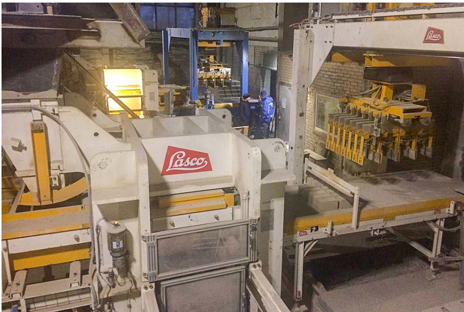
Life Market's sand-lime block plant currently produces around three million blocks per month with three sand-lime block lines from LASCO.
